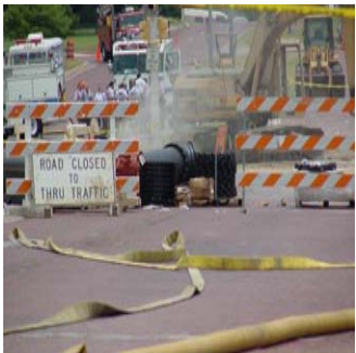
Gas Leak: Result of Construction Efforts
